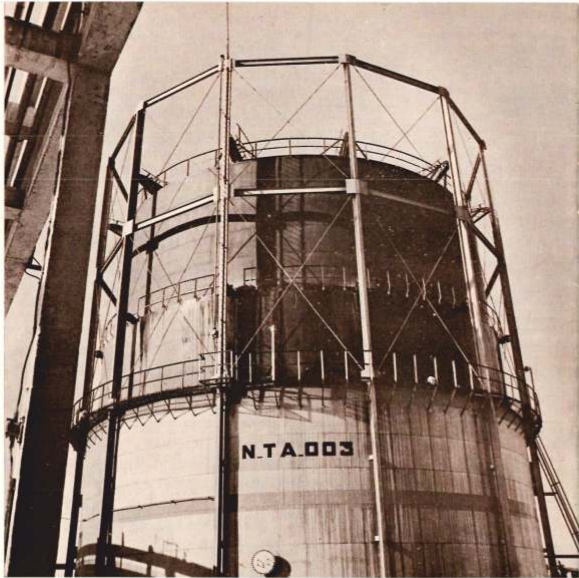
Double lift gas holder for Plastic Resins & Chemicals
